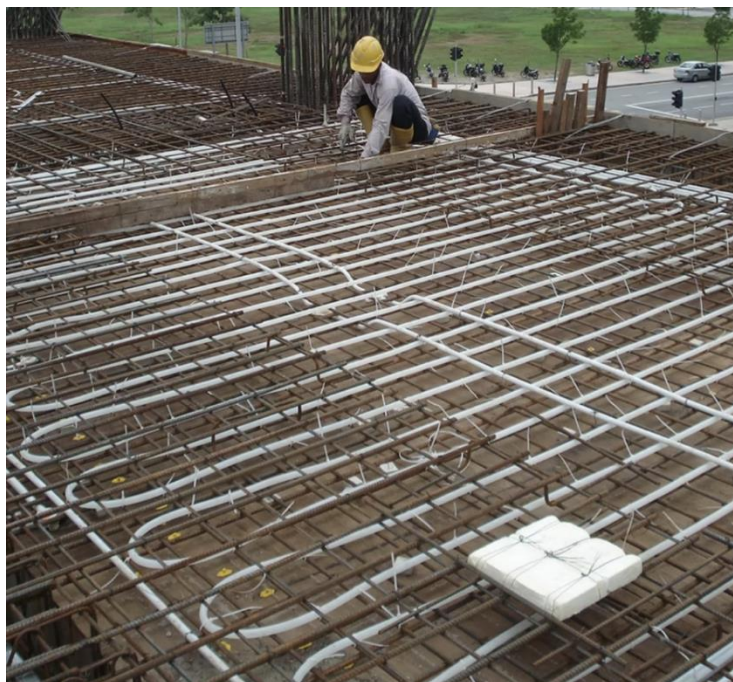
Figure 7. Floor slab cooling system (Photo credit: Original)
