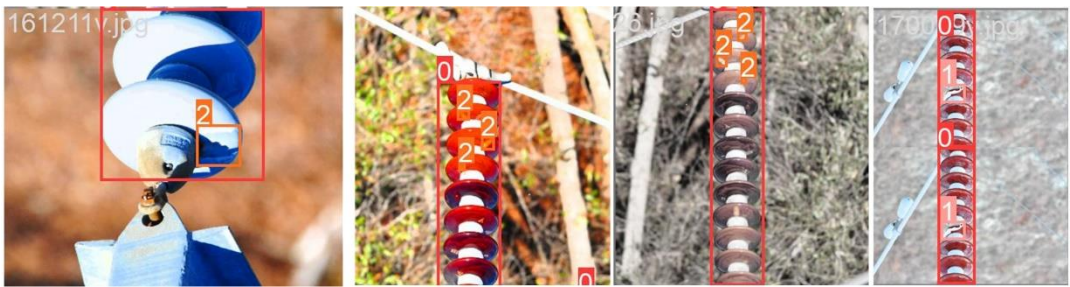
Figure 5. Insulator Defect Recognition Results
